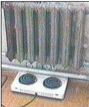
Defrosting a frozen radiator : Cold comfort from frozen radiators
